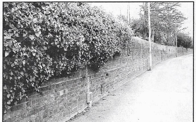
The High Street Wall. An important feature of the Amblecote landscape which should be preserved.
